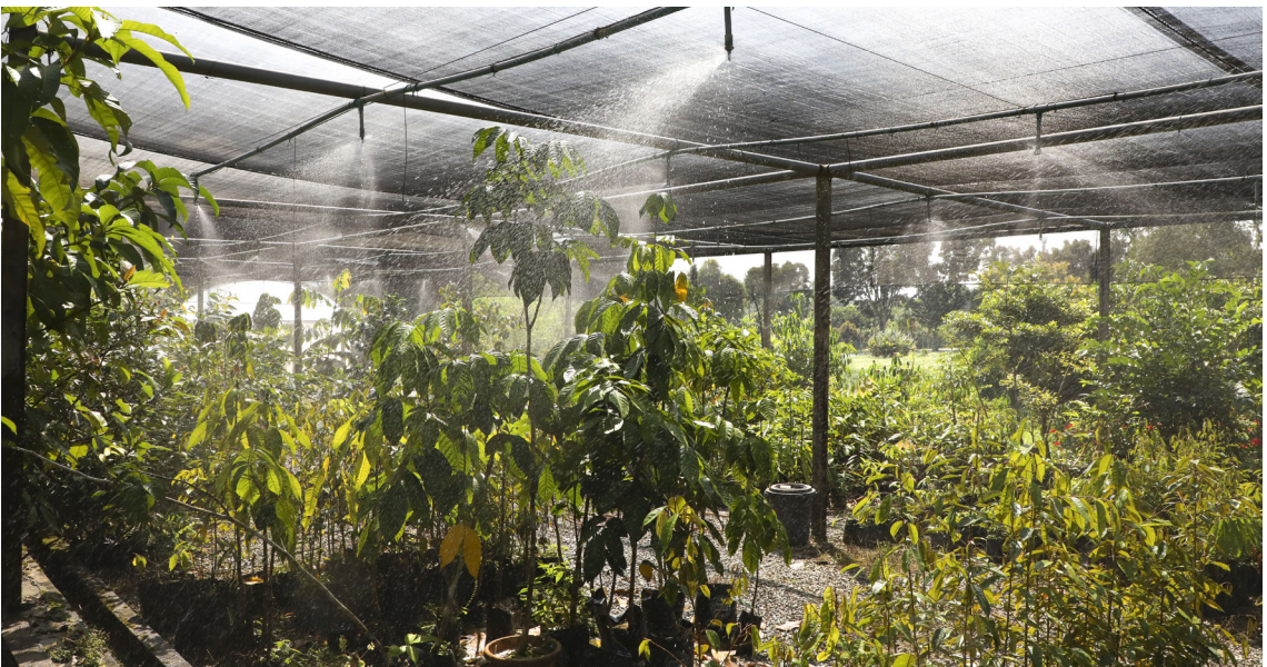
Figure 3.4: Automatic water sprinkler for watering plant
