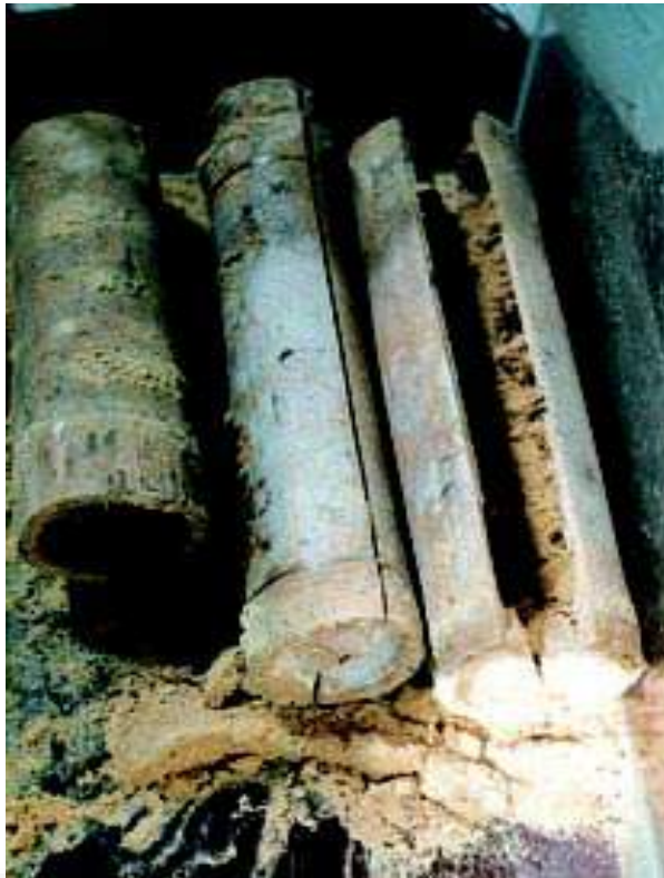
▼ Damage caused by Dinoderus minutus
