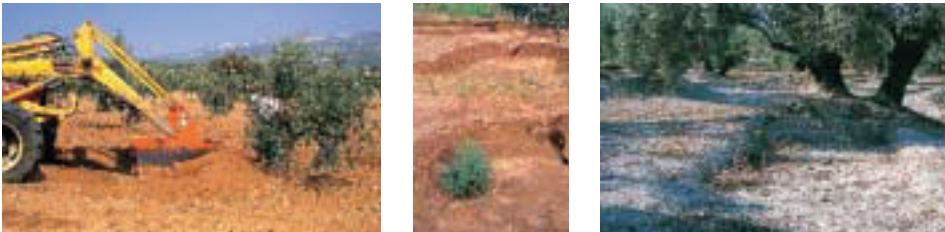
Figure 28. (A) Machine digging small collection pits; (B) pits dug in sandy soil did not take and collapsed easily (C); large, perfectly consolidated pits.
