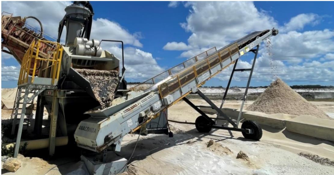
Figure 5 - Third party Sand Wash Plant processing 20-tonne bulk sample from Stockyard Silica Sand Project.
