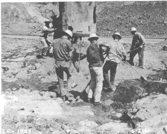
(A) Slurry is spread to fill voids and to smooth irregular bedrock surface...
