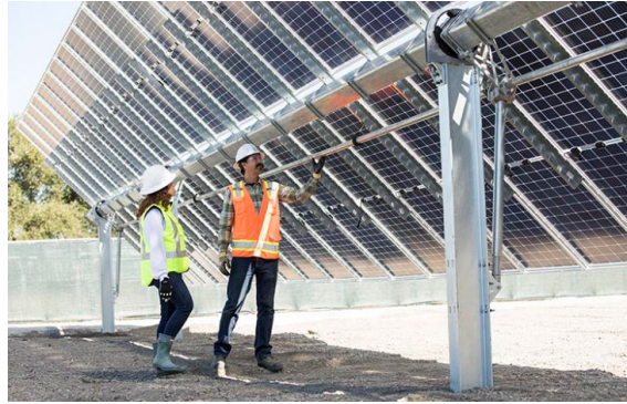
Figure 23: PV tracking system and inverters (Single-axis trackers follow the sun east-to-west on a single point)
