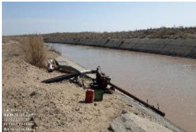
Figure 37: Photo of pump
