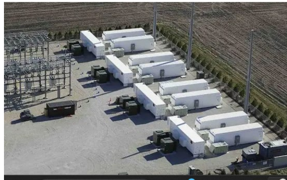
Figure 25: Typical container BESS (external) 9 :
