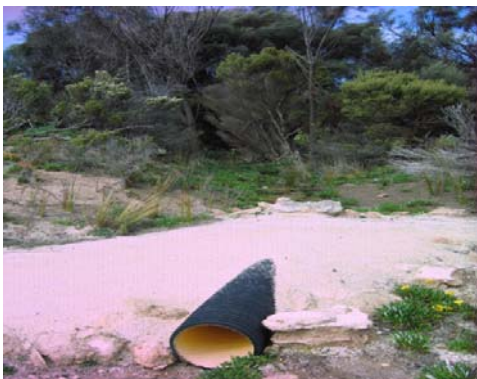
Photo 7—Erosion-prone stormwater outfall
