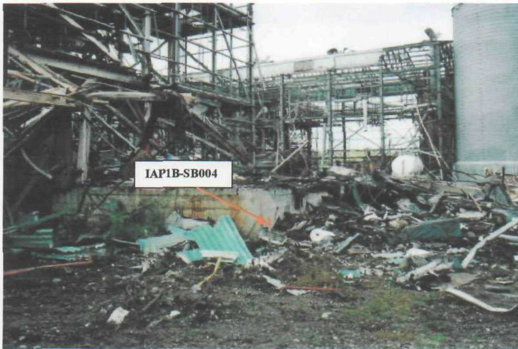
Photo # 4 (Sept. 21, 2000; time: 1446; Roll 1, Sequence 14) Boring Location: IAPIB-SB004 ; South Side of Bld. 415; Facing NW
