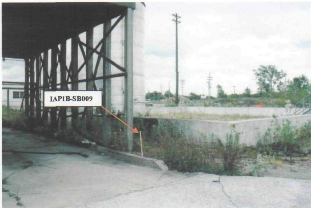
Photo # 9 (Sept. 21, 2000; time: 1453; Roll 1, Sequence 18) Boring Location: IAP1B-SB009 ; SW corner of MDI/TDI Transfer Sta.; Facing SE
