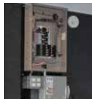
Heavy Duty AC Wiring
