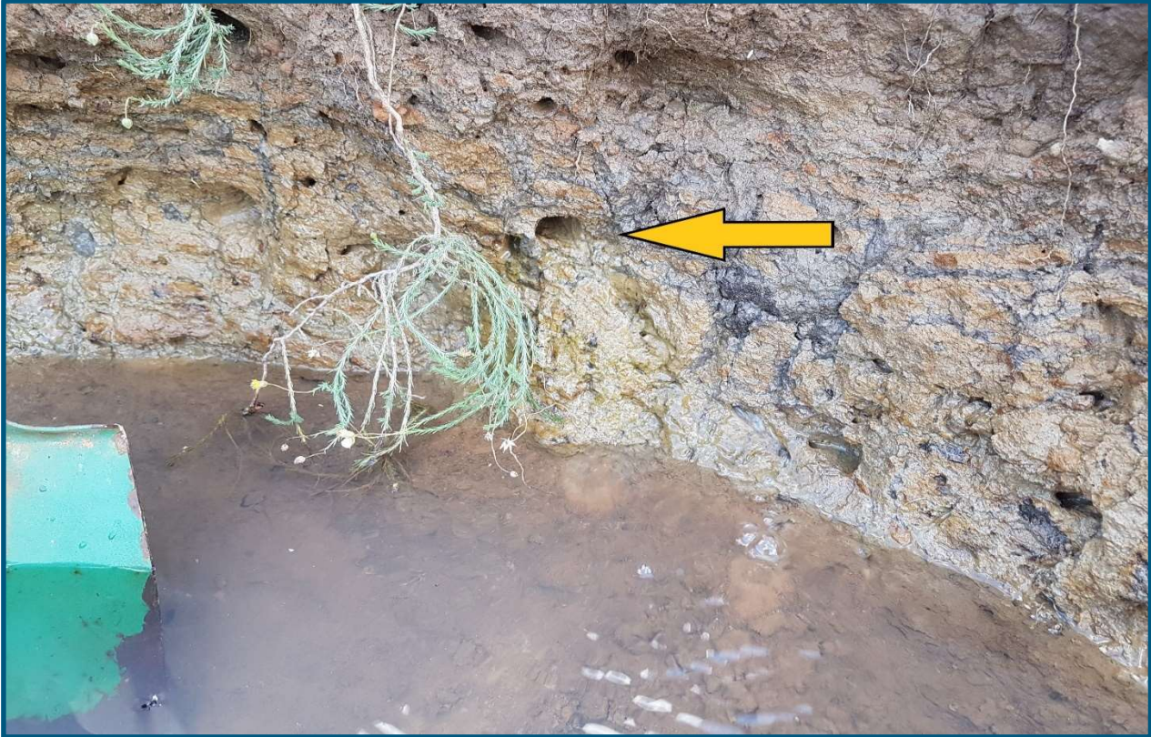
Figure 82: Soil Pipe Exposed by an Active Headcut from Groundwater (interflow)
