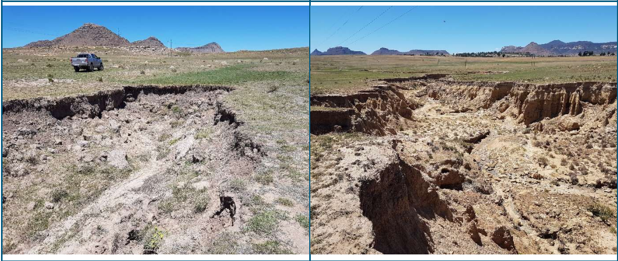
Figure 35: Active Headcut in the Upper Part of Wetland Unit 4
