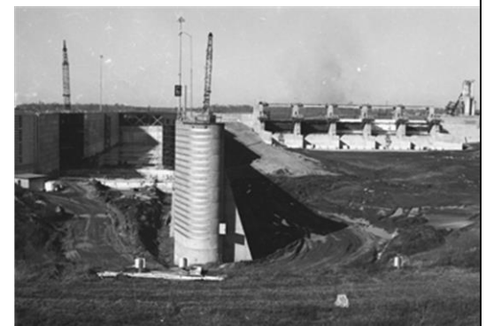
Picture of Columbus Lock and Dam under construction behind where the Plymouth Bluff Environmental Education Center is today. Taken from below the dam which is in the waterway today. Photo by J. Guyton 1978.
