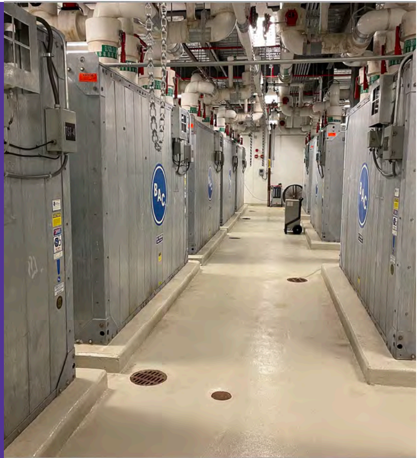
Ice Thermal Storage Tanks Bioscience Plant Germantown Campus
