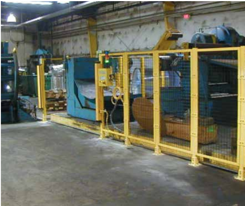
Perimeter guarding system to guard aluminum coil slitting line.
