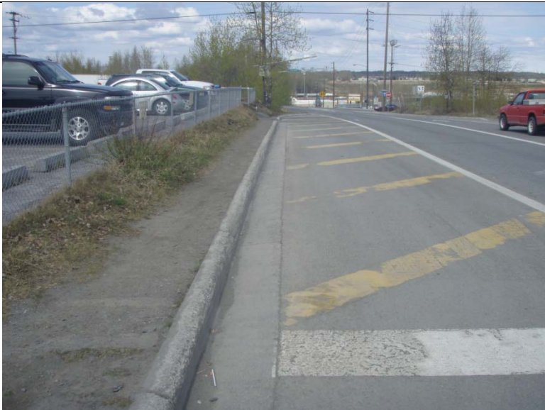
West Side of Ingra St. between 3 rd and 4 th Aves. where new curb and gutter are proposed.
