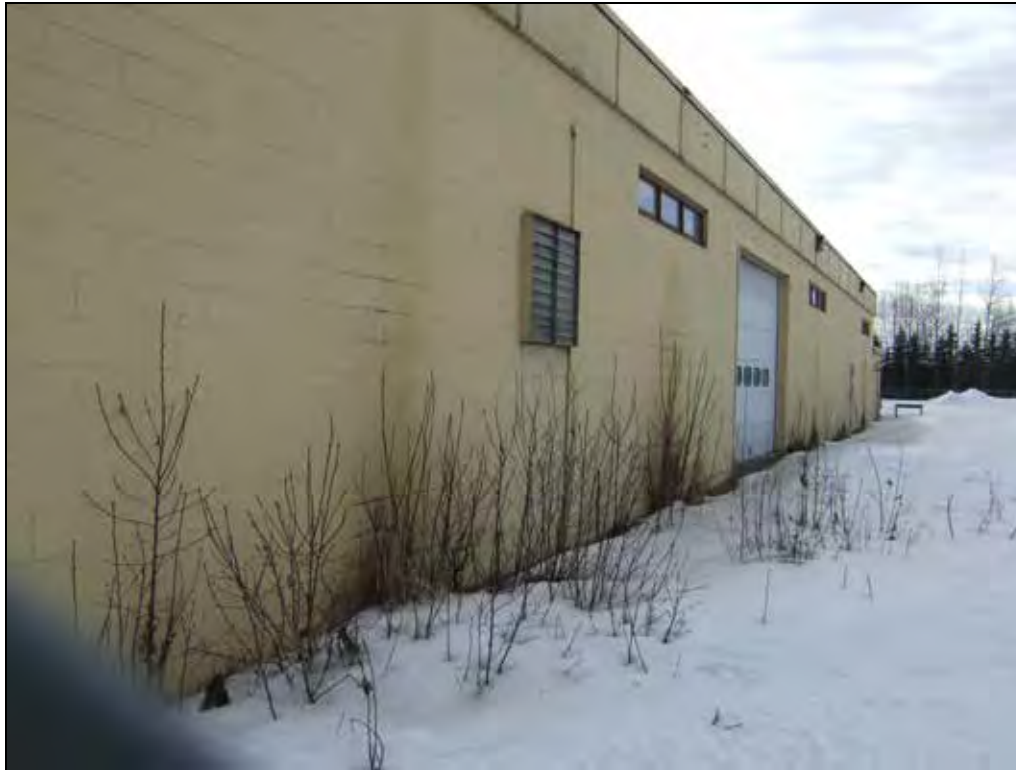
Site ANC-03464, Alaska National Guard Vehicle Maintenance 4902 Spenard Road, Anchorage Alaska Southwest façade, close-up (Jewel Lake Rd 3-16-2011/024)
