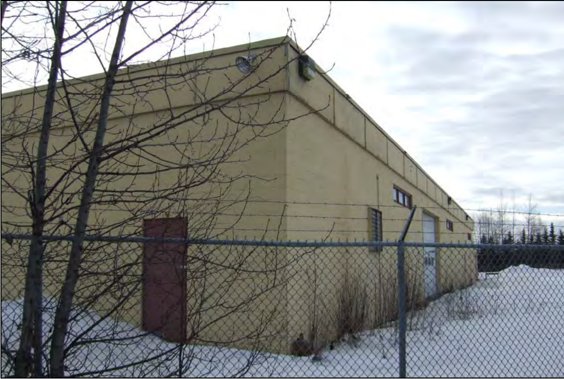
Figure 7.6. Northwest and southwest façades of 4902 Spenard Road, National Guard Vehicle Maintenance Building, view to south.
