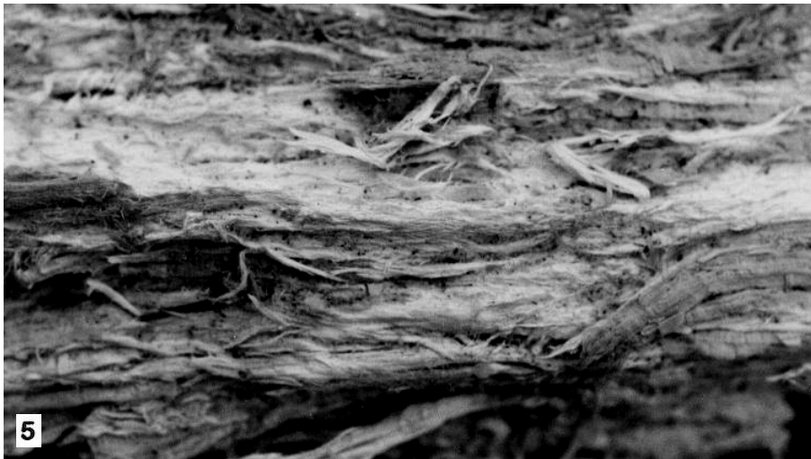
Fig.3. Cubic rot or Brown rot due to Serpula lacrymans . Fig.4. Micro-cubic rot due to Coniophora puteana . Fig.5. Fibrous rot or White rot due to Donkioporia expansa .
