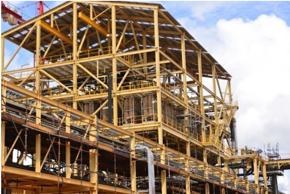
Figure 2.4: The Kwale Mine's Wet Concentrator Plant (WCP)
