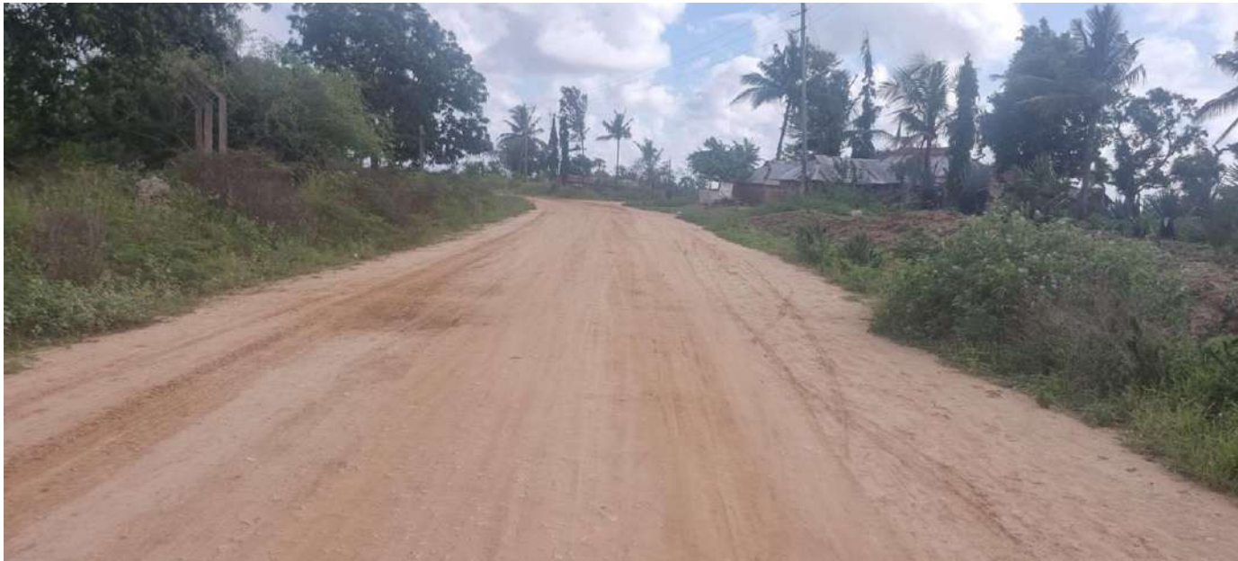
Plate 2.1: The murrum surface access road to MSEZ will be upgraded to better grade murrum standard
