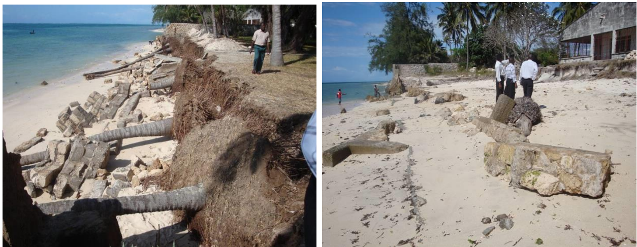
Plate 3.3 Shoreline erosion triggered by shoreline encroachment at Shelly beach, Likoni, Mombasa (Photo credit: James Kamula)
