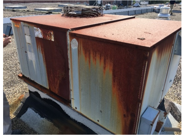
Figure 9. Union High School Rooftop Unit
