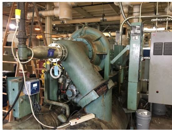
Figure 11. Cooling Tower (top) and Chiller (bottom) at Hannah Caldwell are overdue for replacement
