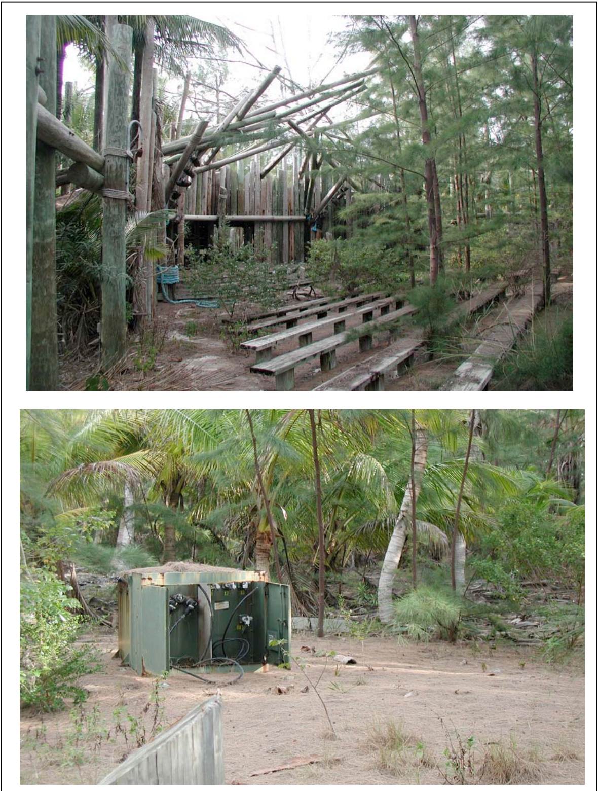
Figure 5.1: Photographs illustrating the clean up needed at the abandoned cruise ship resort site (Disney Treasure Island area). Photo above is 500-seat amphitheatre, below is transformer.]
