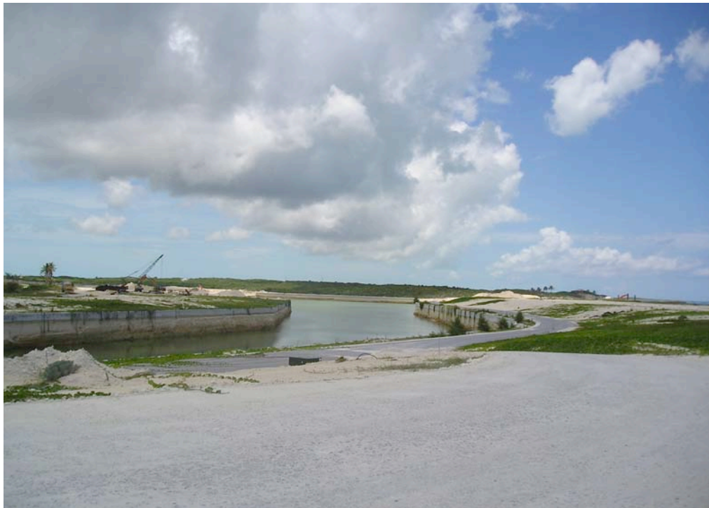
Large-scale marina construction can be incredibly destructive to land and sea environments. Special care must be taken to avoid high turbidity (top photo) and Erosion (lower photo). (Photos taken at Four Seasons, Exuma).
