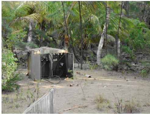
This is a transformer from the former Disney development which will need remediation and removal
