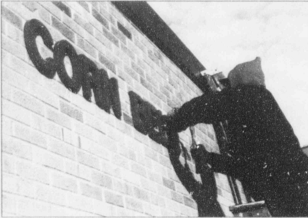
At left, a new sign is installed on the front of Corn Belt Power headquarters building that will match the new dark green pitched roof. Construction of the roof began in late 1993.
