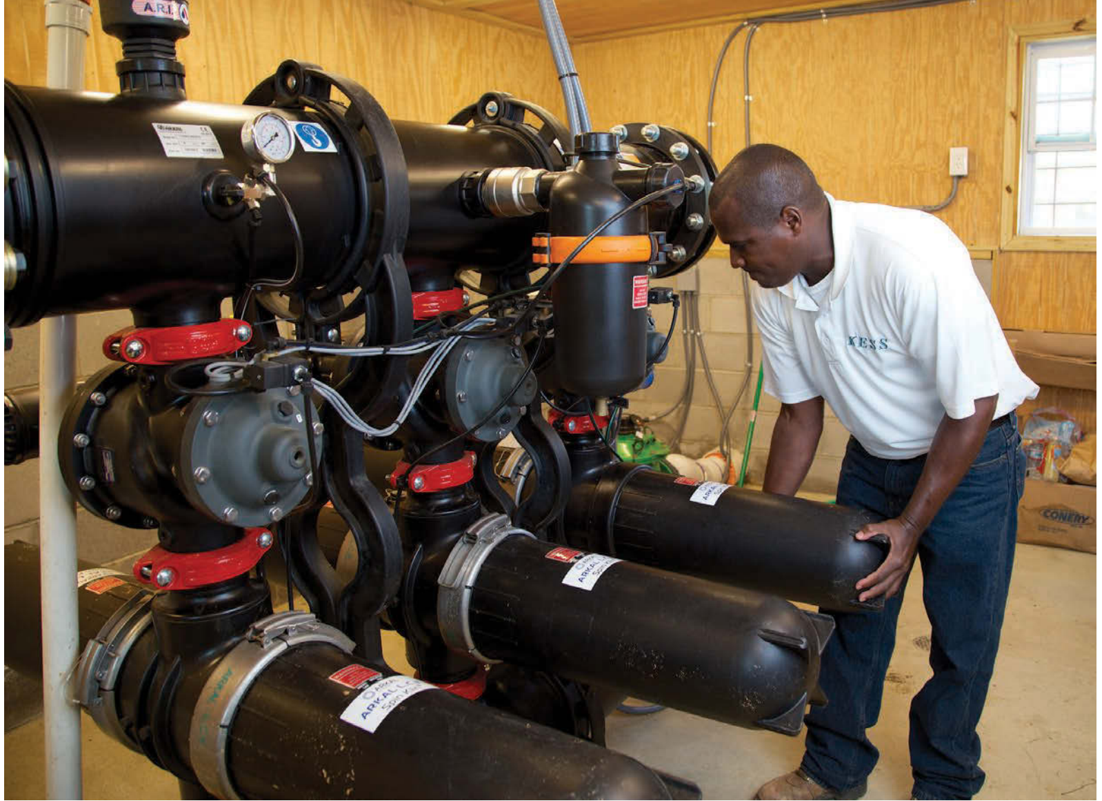
Sears Smith removes a cover from an Arkal Filtration Systems filter at a KESS Environmental Services facility for The Waters development.
