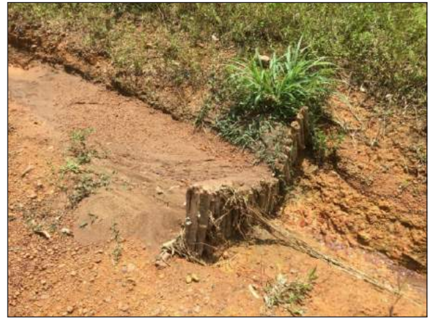
Figure C.6.14: Scour check made from wooden stakes
