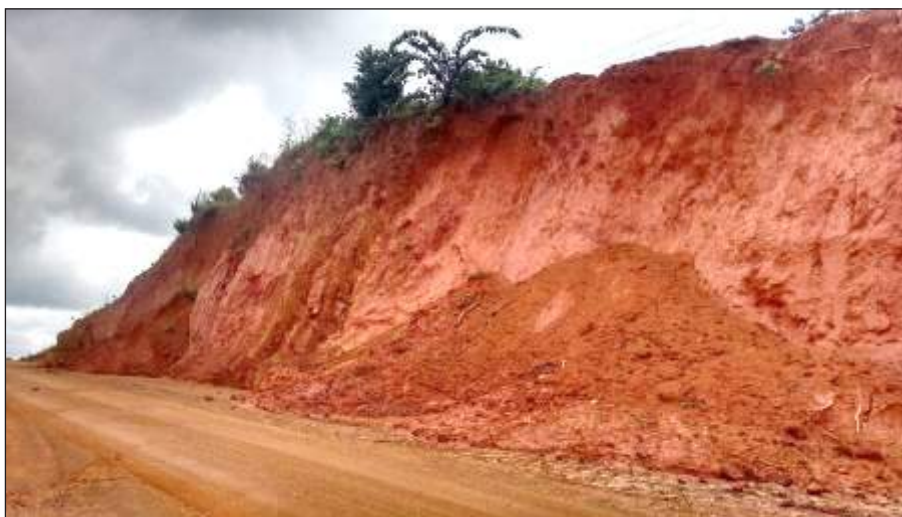
Figure C.7.3: Failure of the upper portion of the cut slope in the weathered mantle
