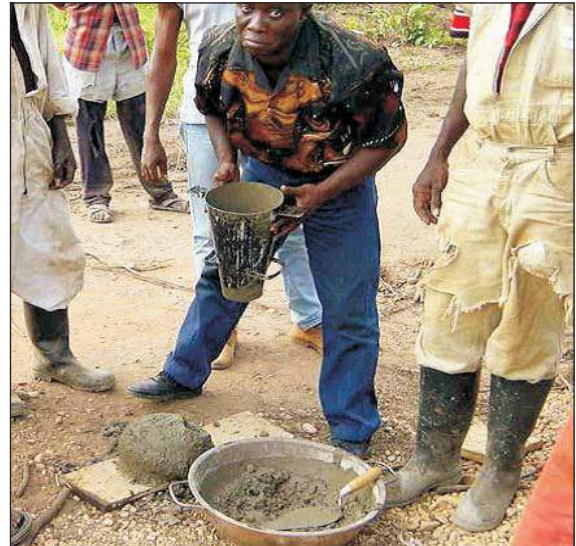
Figure C.8.11: Collapsed slump - too much water
