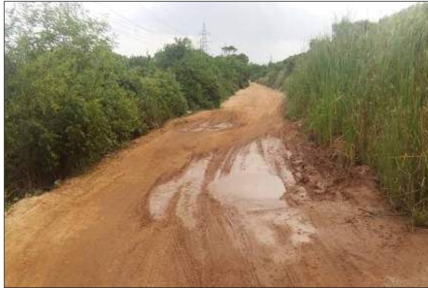
Figure C.9.2: Stagnant water due to poor camber
