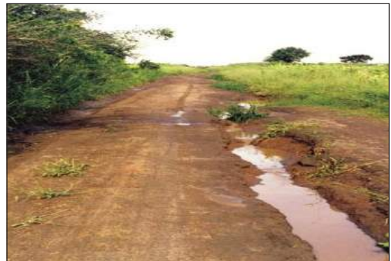
Figure C.4.15: Poor drainage on flat ground
