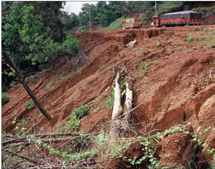
Figure C.7.12: Severe erosion of embankment material
