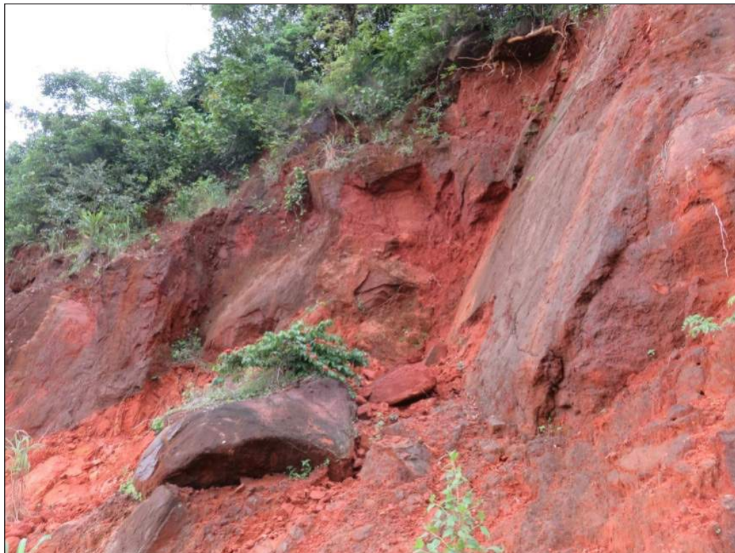
Figure C.7.1: Shallow slide in roadside cut slope
