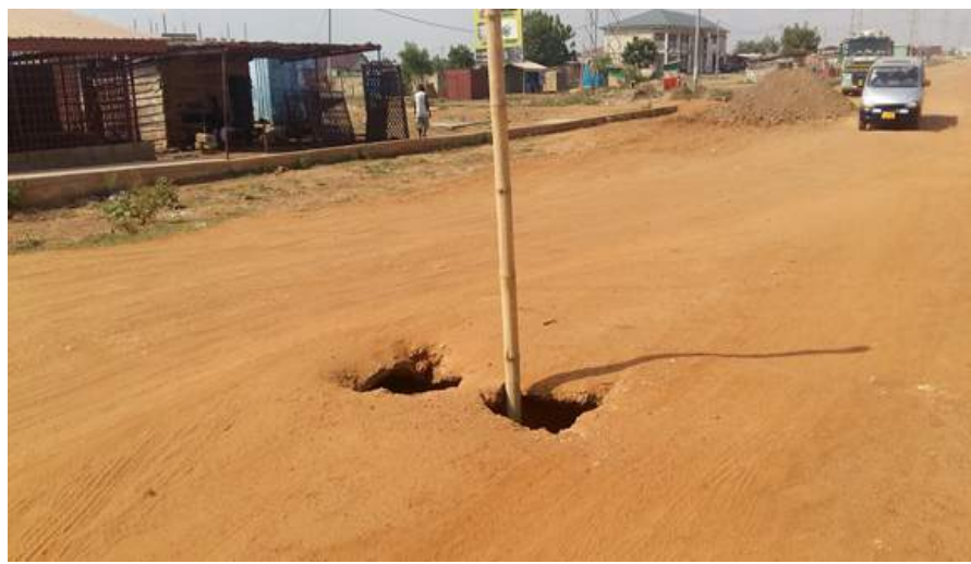
Figure C.4.8: Damage to pipe culvert due to inadequate cover
