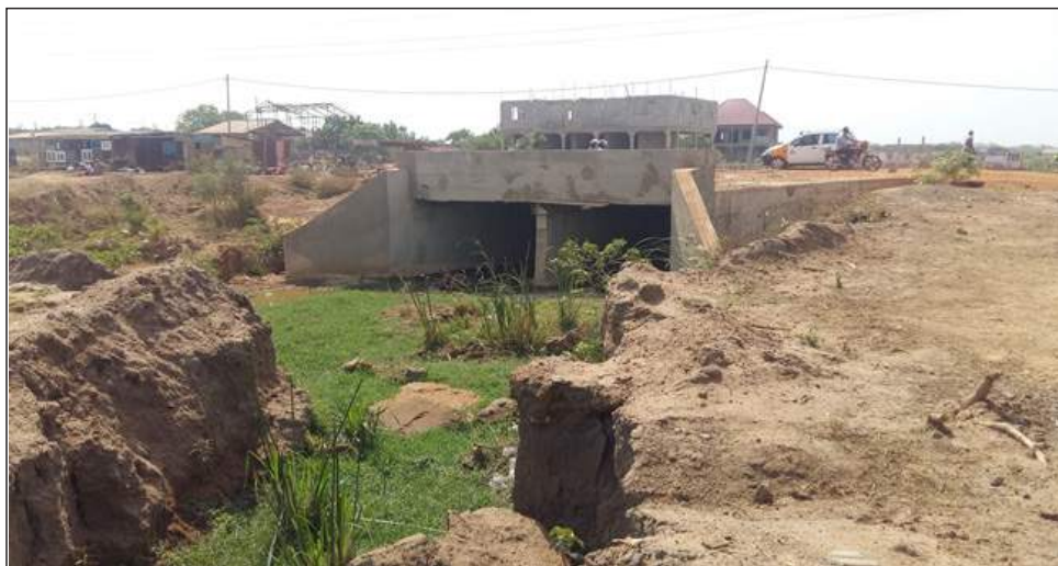
Figure C.6.7: Erosion of channel downstream of culvert
