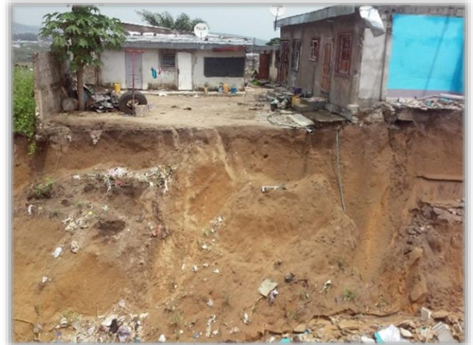
Figure 2 : Destruction of a plot in the Makabandilou district
