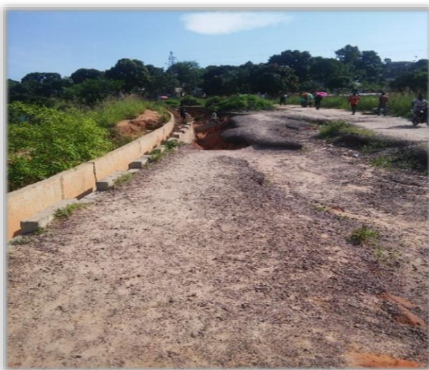
Figure 1 : View of erosions in the Lebled district
