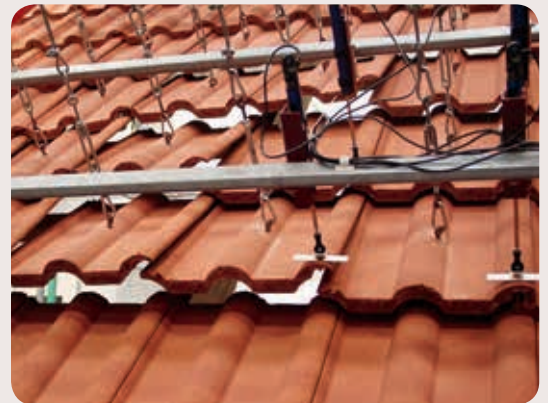
REDLAND SEVERE LOAD TESTING FACILITY
