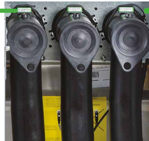
TH110 mounted on cable termination
