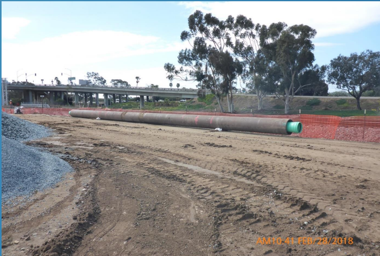
False Bay Trunk Sewer at Knoxville – 30-inch Steel Casing
