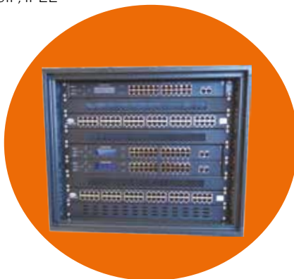
INSTRUMENT ROOM 9U PHONTECH SYSTEM CABINET
