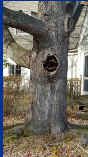
Figure 1 — Methods by which decay enters a tree. From Pathology of Trees and Shrubs, by T. B. Peck, with copyright permission from the publisher.
