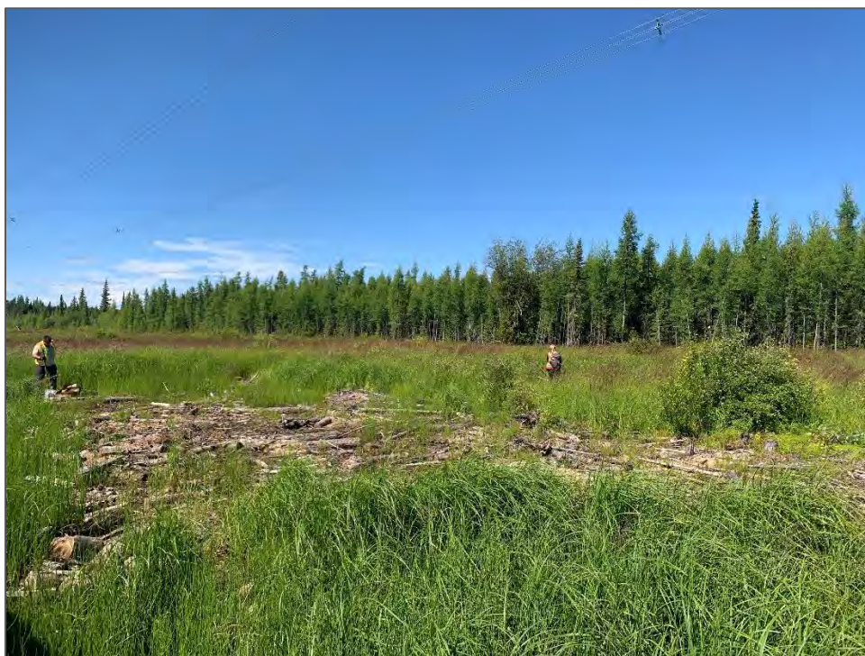
Plate 3.3-3. Wb06 Tamarack - Water sedge - Fen moss bog at wetland WL115 in 2020 showing the cleared and grubbed portion within the transmission line right-of-way.
