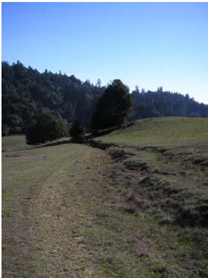
Photopoint 78. Erosion along road-gully 11.
