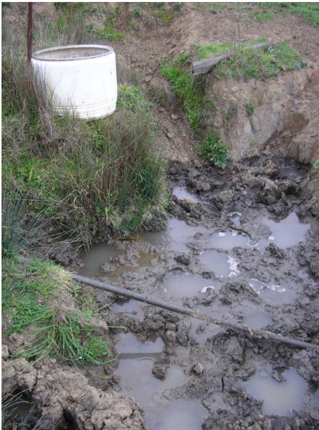
Spring requiring repairs
