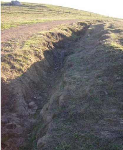
Photopoint 92. Erosion along road.
