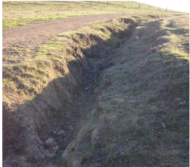
Erosion along Wright Hill Road
