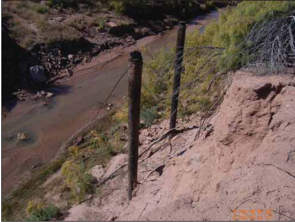
Figure 4.11. Wooden pilings eroding out of northern bank, facing southwest.
