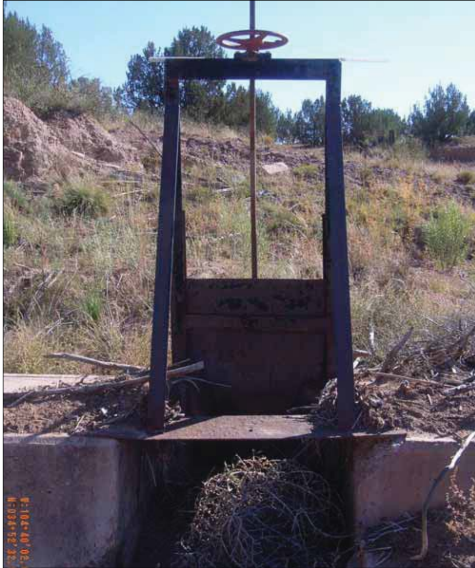
Figure 4.31. Sliding metal outfall gate with screw-type mechanism, situated at eastern end of spillway.
