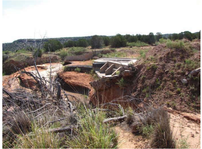
Washed out West Puerto de Luna diversion dam on Agua Negra Creek, looking downstream and to the east.
