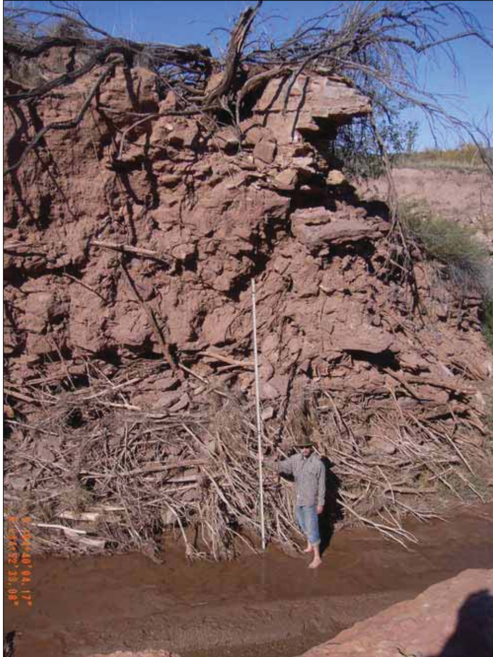
Figure 4.45. Another view of the northern cross-section of the diversion dam, facing northeast. Note remnants of masonry wall visible in cross-section.
