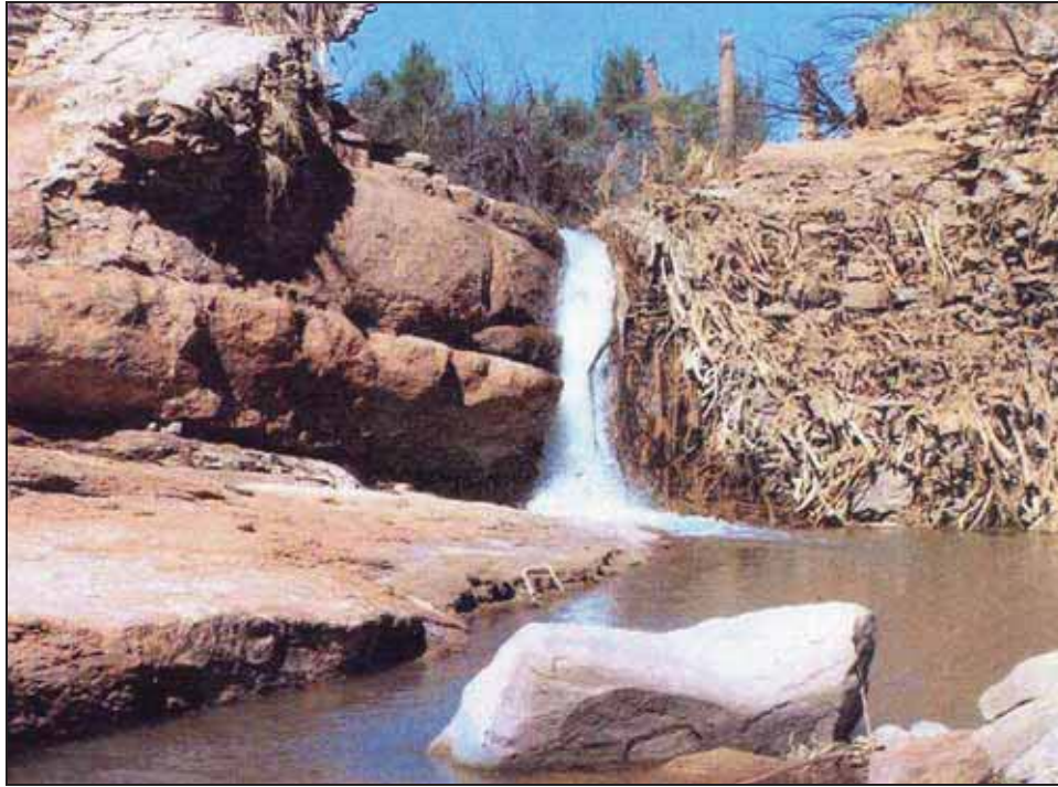
Figure 4.17. View of the diversion dam after the initial 2005 breach, facing west. Note wooden pilings visible over the top left.
