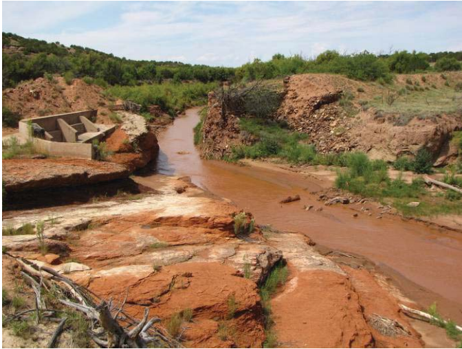
Washed-out West Puerto de Luna diversion dam on Agua Negra Creek, looking upstream and to the west.
