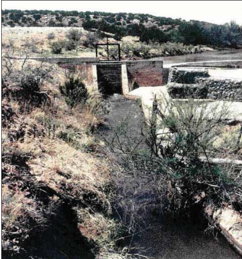
Figure 4.39. Headgate and acequia before breach, facing west. (Photograph courtesy of the West Puerto de Luna Acequia Association).
