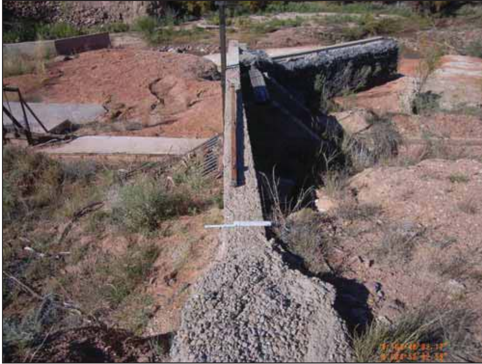
Figure 4.37. View of the headgate structure from the south, showing concrete wall and gabion.
