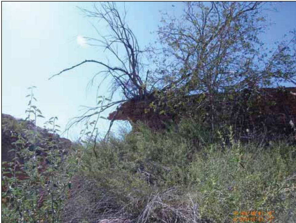
Figure 4.51. Northern segment of masonry diversion wall, facing west, showing remnant portion overhanging the breached diversion.
