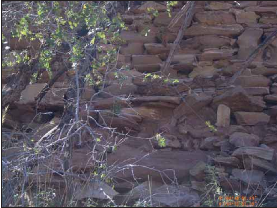
Figure 4.53. Base of masonry diversion wall, facing west, showing transition to rubble bank armoring.
