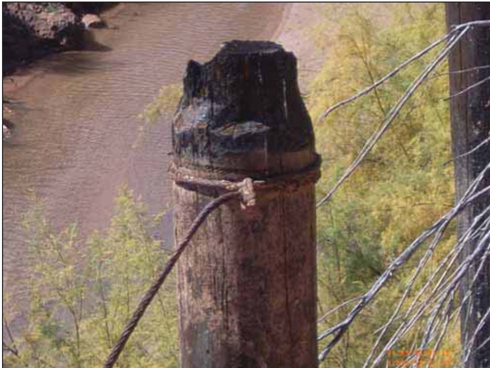
Figure 4.12. Top of one of the wooden pilings eroding out of the south bank, showing attached steel cable, facing west. Dangling cable end points southeast.
