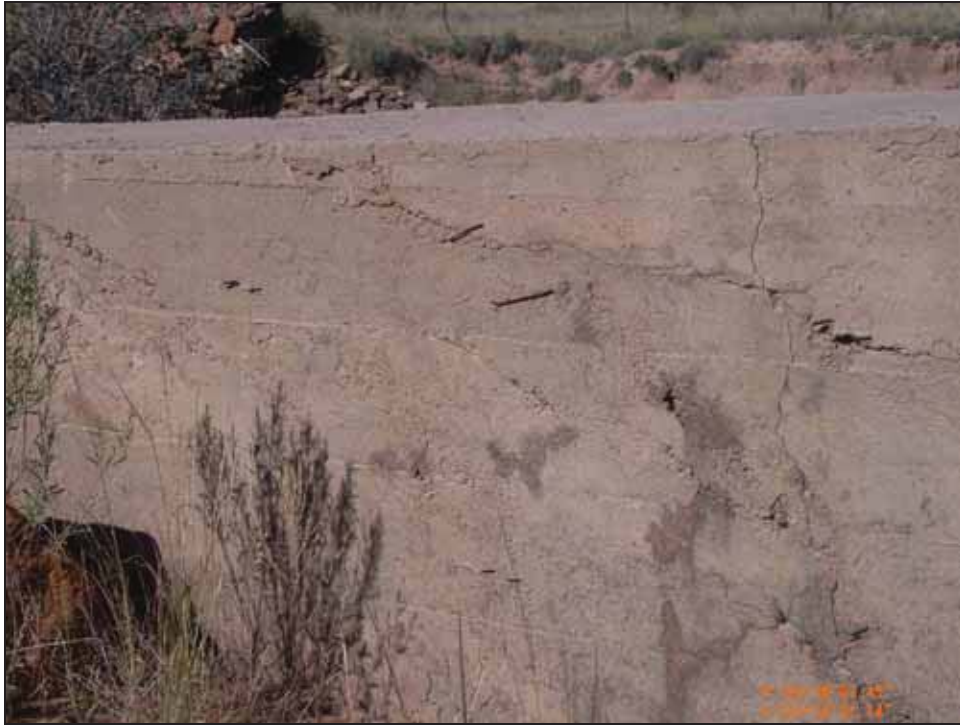
Figure 4.26. Southern face of the masonry spillway wall, facing north, showing wire used to reinforce concrete plastering covering wall face. Note also multiple patching / plastering events visible on this wall face.
