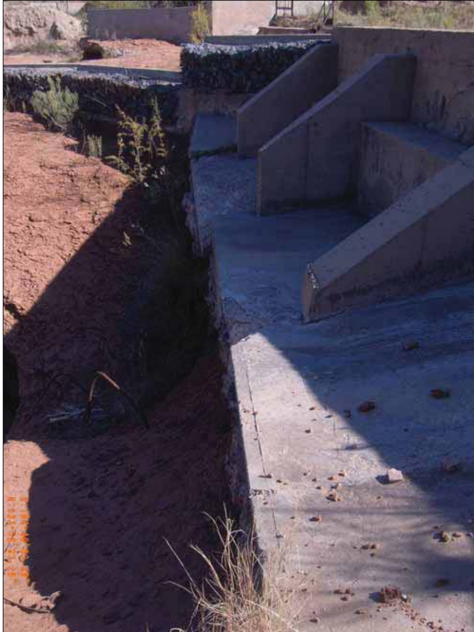
Figure 4.29. View of wall at north end of spillway, with gabion in background.
