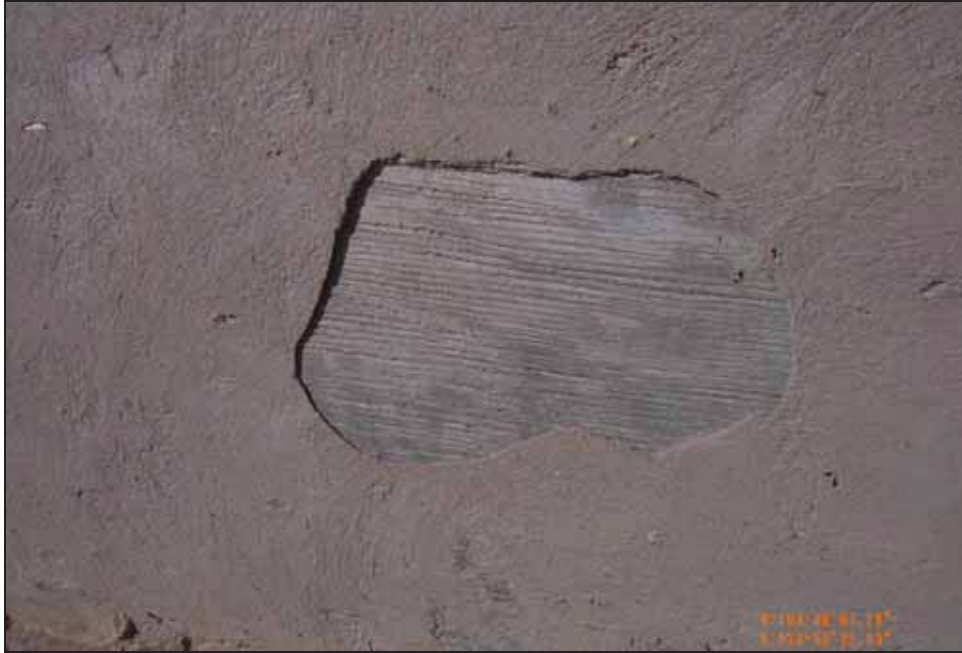
Figure 4.27. Close-up of hole in concrete plaster, showing different concrete surface underneath.
