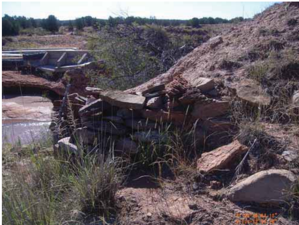
Figure 4.7. Northern end of eastern retaining wall, arcing inward toward the earthen berm.
