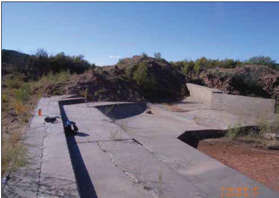
Figure 4.22. View of southern portion of spillway, facing west. Note recent bulldozed rock / dirt pile covering the spillway's western edge.
