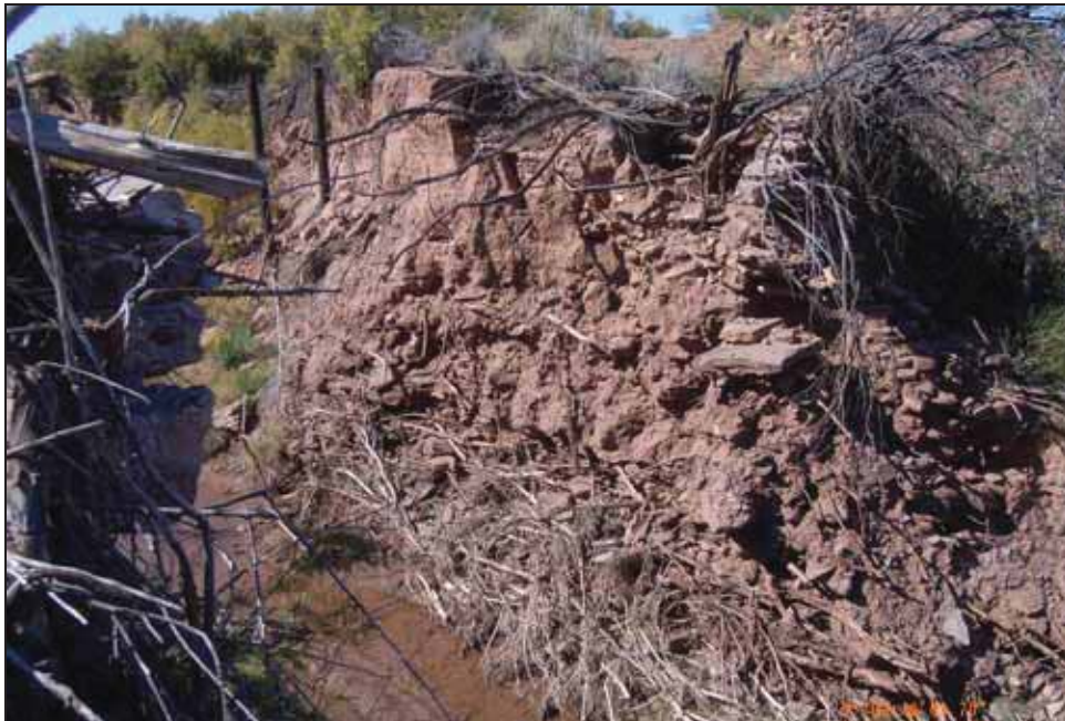
Figure 4.43. Northern cross-section of diversion dam, showing successive layers of rock and brush, facing northwest.
