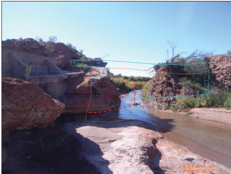
Figure 4.56. Approximate extrapolated positions of bedrock (dotted line), masonry wall (blue), and rubble armoring (orange).
