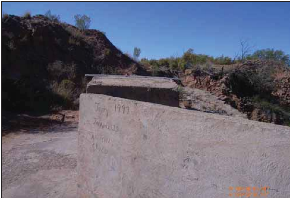
Figure 4.28. End-on view of masonry/concrete spillway wall, facing west, showing wall with gabion in foreground.
