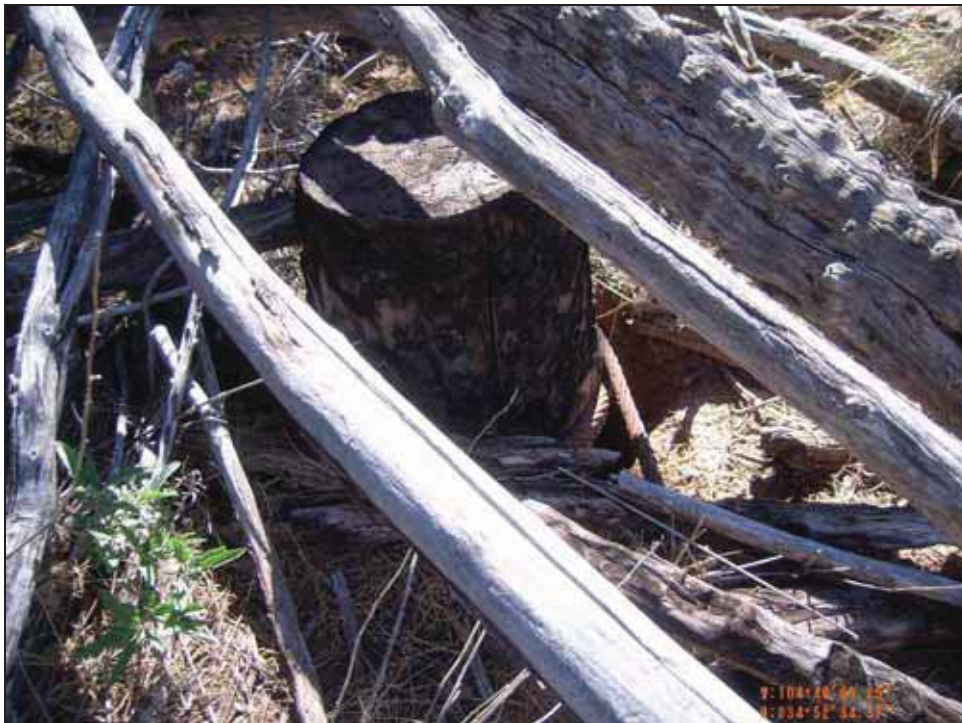
Figure 4.14. Another wooden piling protruding approximately one foot above current ground surface. Note steel cable wrapped around it.
