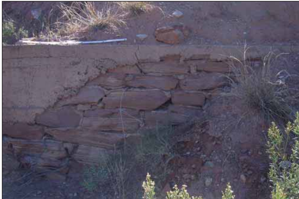
Figure 4.25. Eastern portion of northern spillway wall, showing original sandstone masonry visible under fragmented concrete plaster. Folding ruler at top left is one meter in length.
