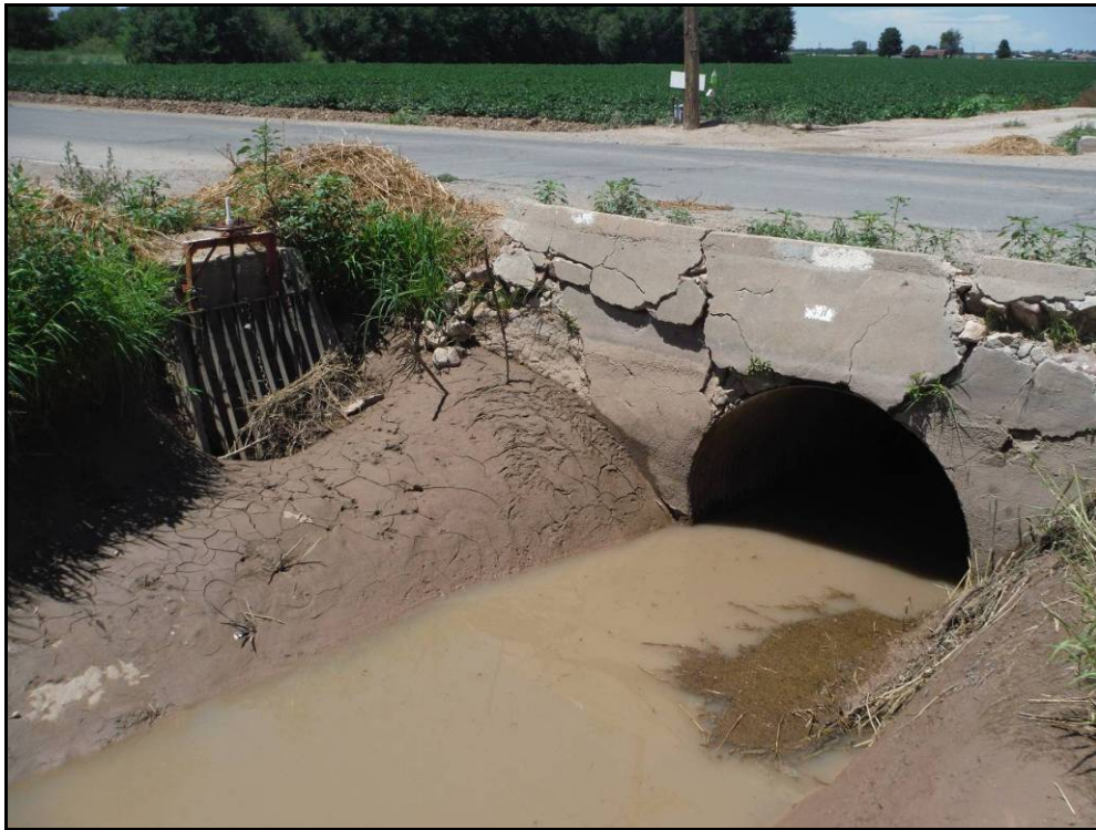
Figure 5. Canutillo Lateral on Borderland Road, near the Rio Grande Bridge, facing north.
