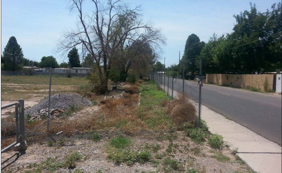
Roadside drainage ditch (D-106) located along Bosque Road, south of Western Way (Phase II survey area). Photo Direction: south (downstream). Photo taken 8/18/2015.
