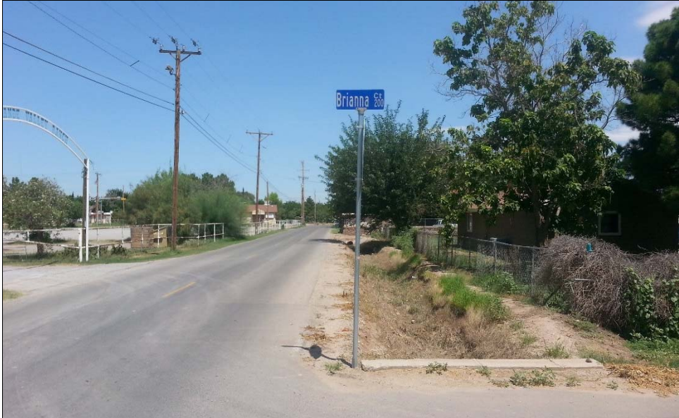
Beginning of Phase II survey area. Roadside drainage ditch (D-107) located north of Brianna Court. Photo Direction: north (upstream). Photo taken 8/18/2015.
