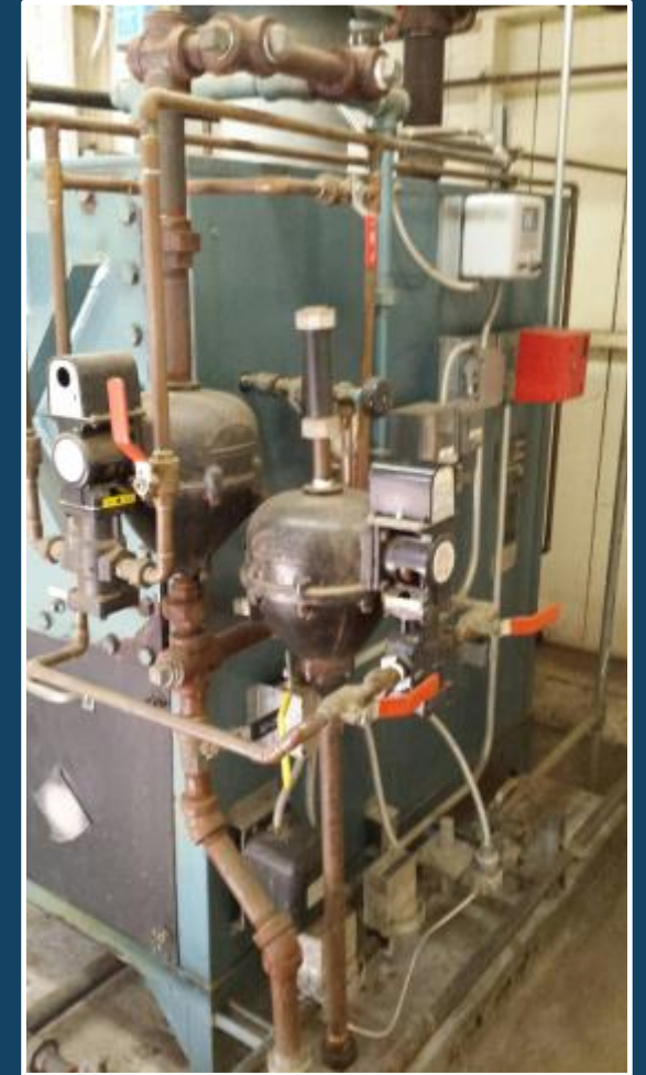
Boiler used to generate steam
