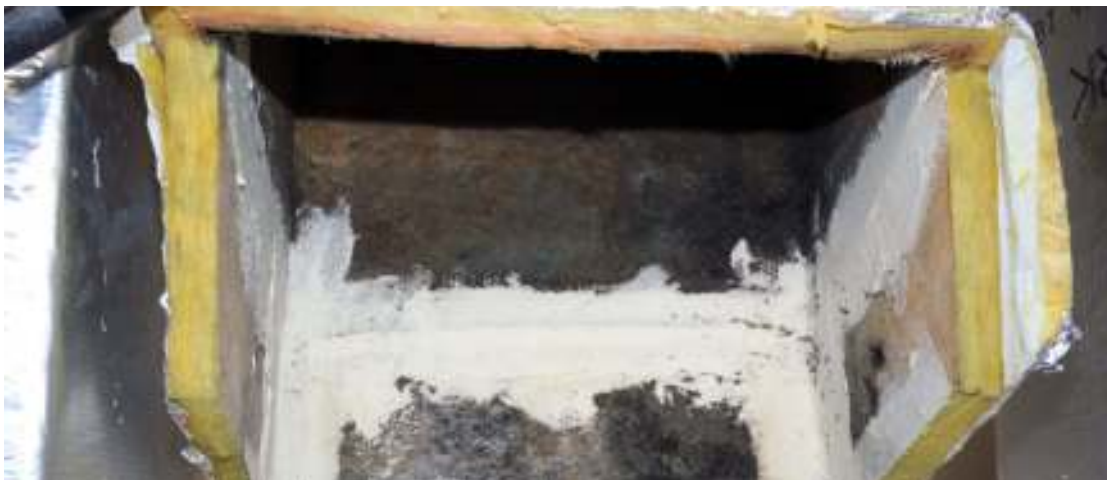
AC supply plenum full of toxic mold.
