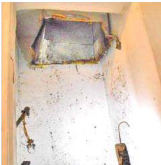
Mold hidden behind air handler.
