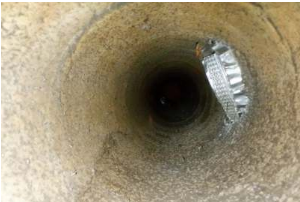
Nasty AC ducting. Clean or replace.
