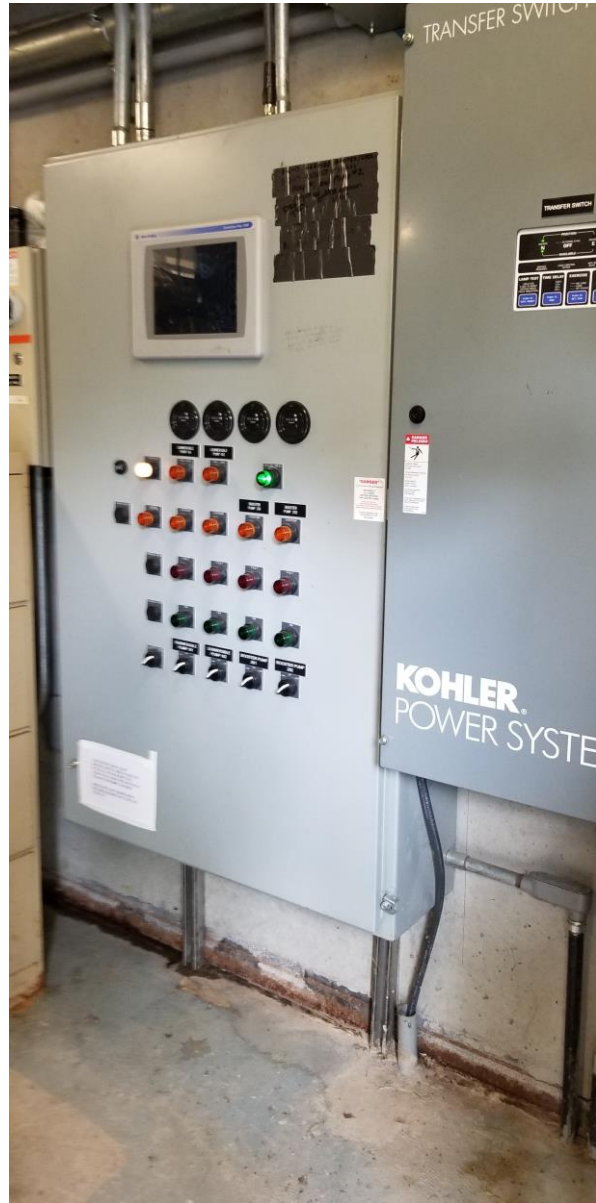
Figure 3-5: Interior of Existing Scott Road Pump Station, Control Equipment
