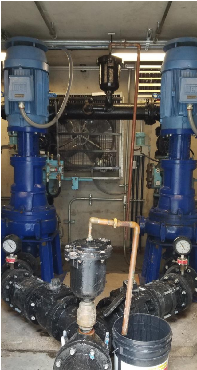
Figure 3-4: Interior of Existing Scott Road Pump Station, Dry-Pit Pumps
