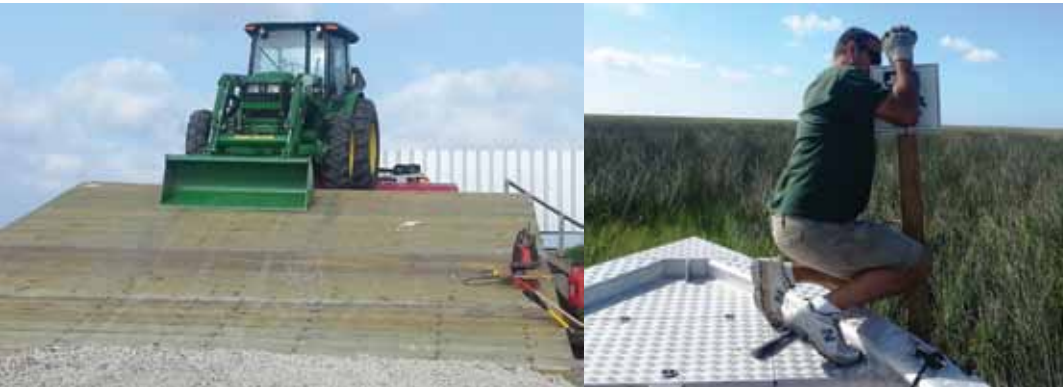
LEFT: Completed storm platform on the Big Impoundment to store equipment. RIGHT: Staff posting boundary. (Marsh Island Refuge)
