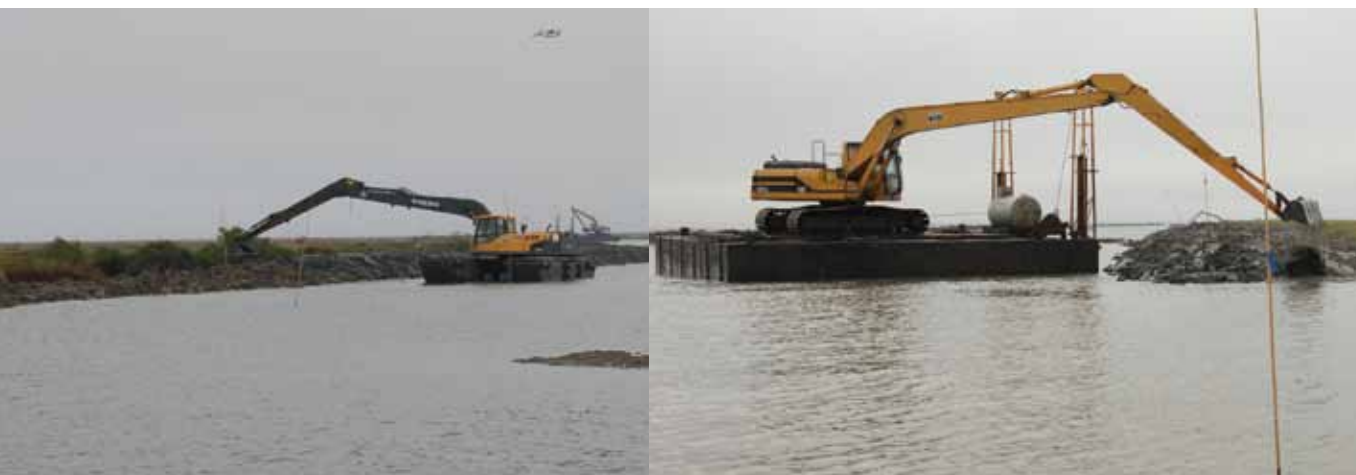
TLCD Terrace Projects in the PAC/DU management unit parallel to the PAC/DU levee. LEFT: TLCD amphibious excavator building terraces. RIGHT: Contractor (Lowland Const.) building terraces via "flexi-float" and land based excavator. (Pointe-aux-Chenes WMA)
