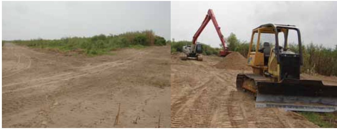
LEFT: New roads/hunting lanes installed on reservoir. RIGHT: Staff enlarging Loomis Pass campground and repairing hog damage. (Pass-a-Loutre WMA)
