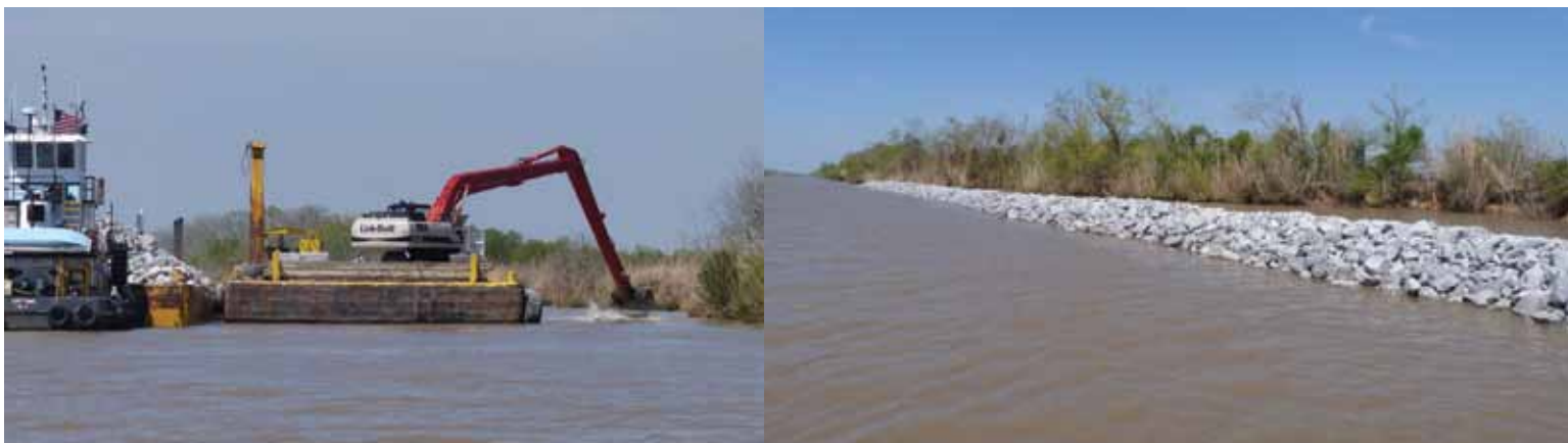
LEFT: Placing rock on the Gulf Intracoastal Waterway (GIWW). RIGHT: Rock placement on GIWW completed.
