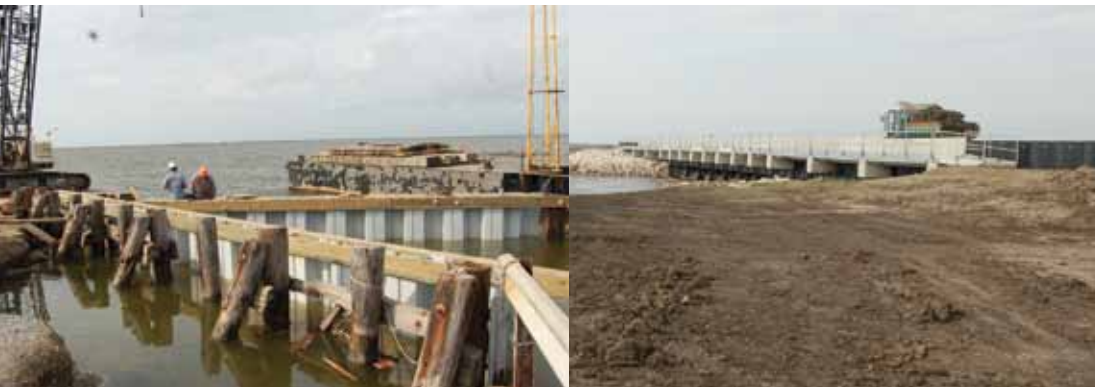
LEFT: Island Road S-1 Structure repair. RIGHT: Completed Bridge on Montegut Unit S-2. (Pointe-aux-Chenes WMA)
