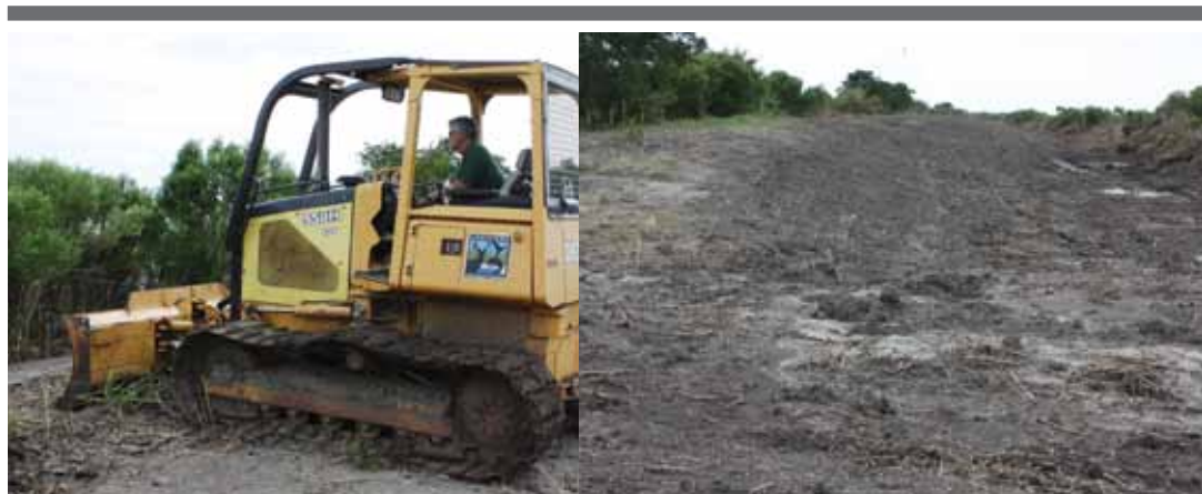
Photos of levee clearing project at Big Impoundment. LEFT: G. Broussard operating bulldozer. RIGHT: Recently cleared levee. (Marsh Island Refuge)
