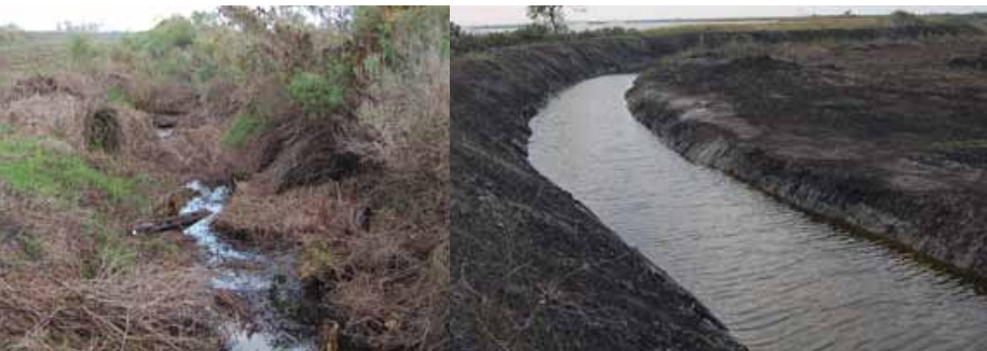
BEFORE & AFTER: Point Farm ditch clean out projects conducted by LDWF staff. (Pointe-aux-Chenes WMA)
