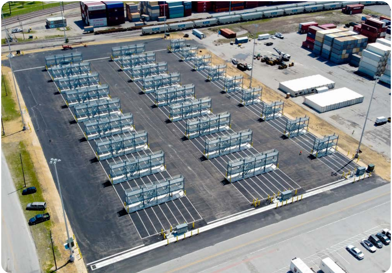
Above: The Port of Wilmington's new refrigerated container yard, completed in April 2020, has increased the Port's refrigerated container ("reefer") plugs from 235 to 775. Phase 2 of the project would allow the Port to expand to over 1,000 plugs. Photo Credit: North Carolina State Ports Authority
