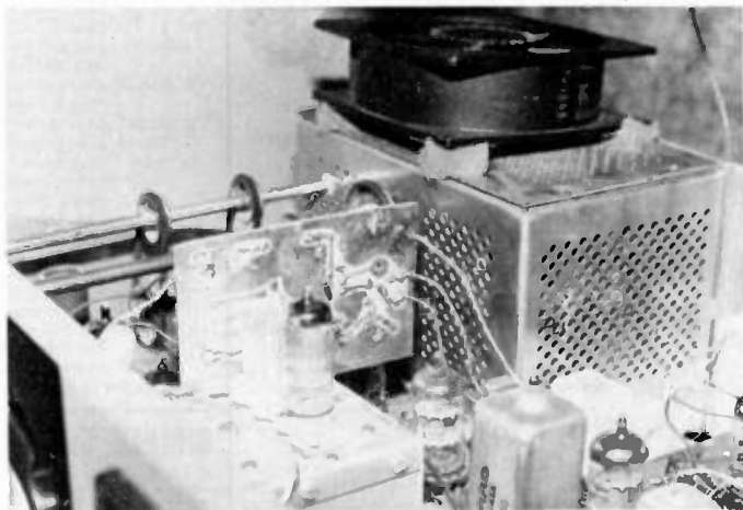
Photo B. Rear view of FSK board showing wires from computer.
