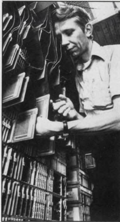
Technician inserts circuit packs in the 1A stored-program control unit of Bell Telephone's 4 ESS for long-distance calls. The hanging cables are connected to test equipment.
