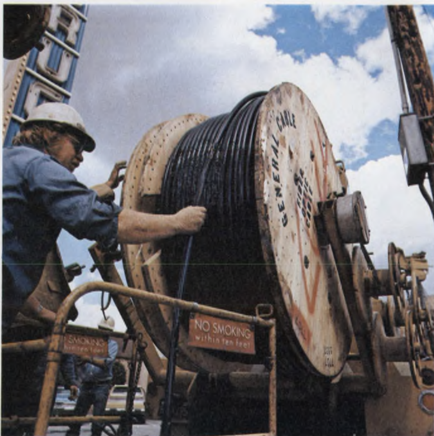
Fiber-optics cable for a 5.6-mile telephone system in California is pulled through an underground conduit. The 1.544-Mbit/s system, developed by General Telephone and Electronics, uses cables by General Cable Corp.
