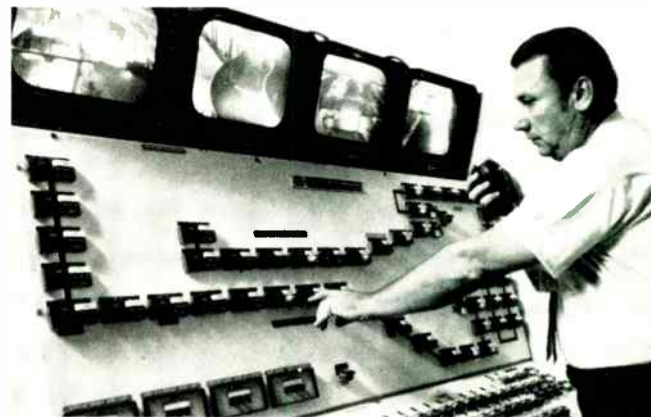
Successful diversification: Aerojet-General's airline baggage system stems from industrial programmable controller capability.
