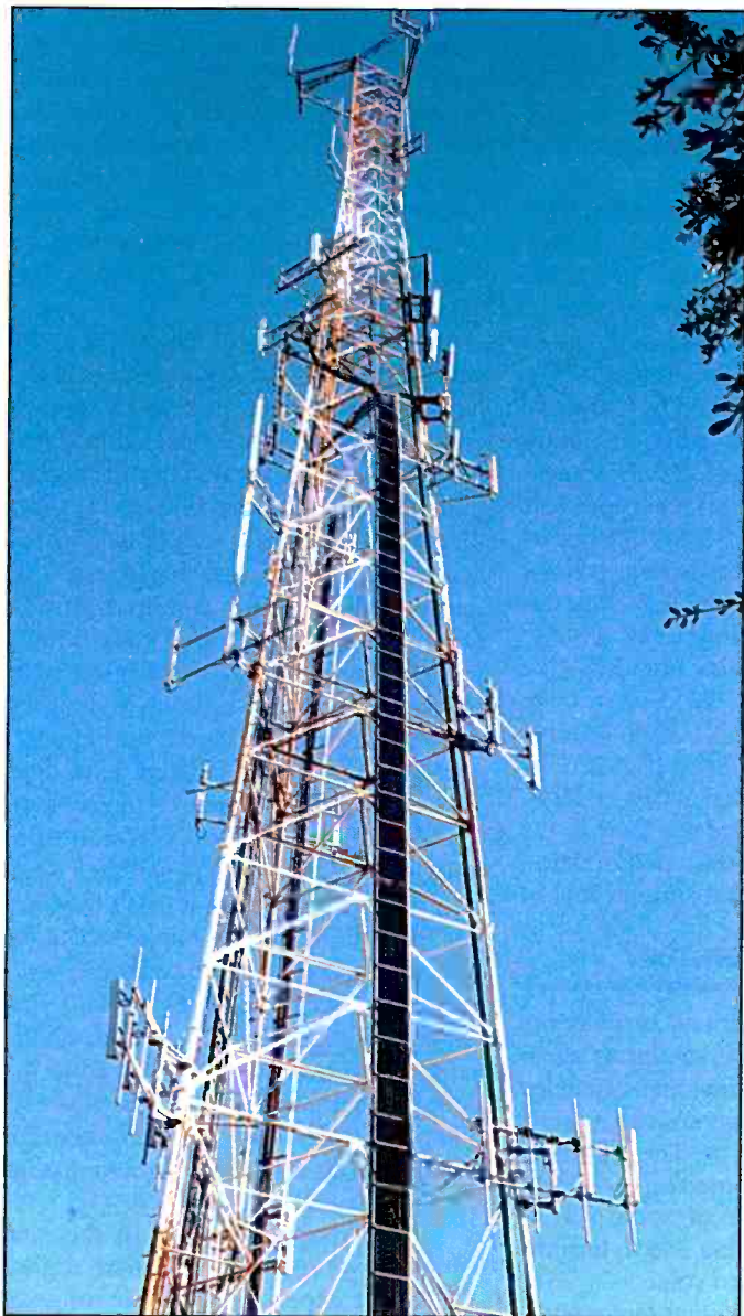
Communications tower in North Arlington on Collins Street.
