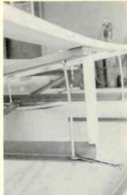
FIG. 9—ADJUSTMENT BOLTS are set for proper spacing between vertical frame rib and wood strip. Here a \frac{7}{4} -inch spacer aids adjustment at 72-inch point.
