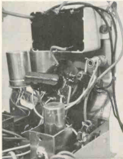
The high-voltage system is mounted vertically on the right side of the main chassis.
