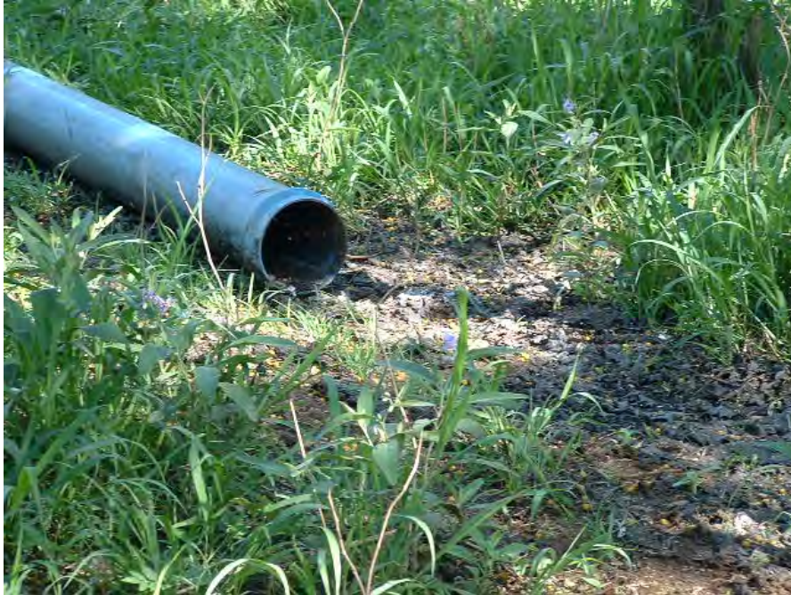
Figure 2.39: Effluent discharge pipe leading onto the banks of the Klein Nyl River (November 2002).
