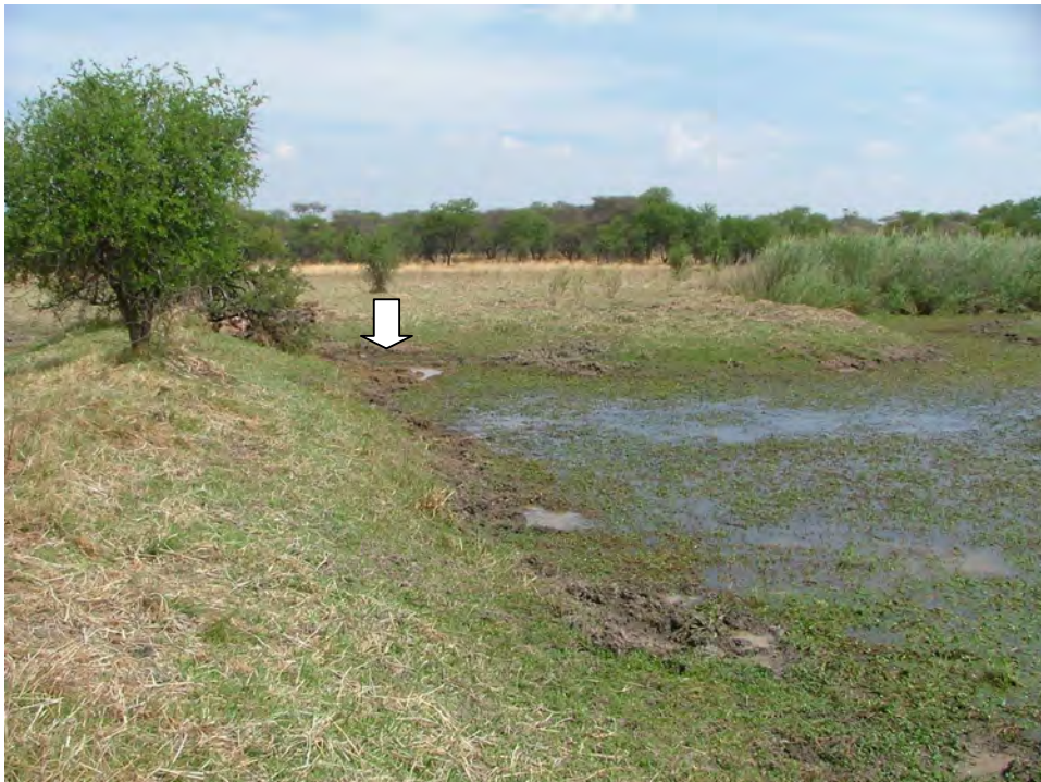
Figure 1.13: A view of the weir during the low flow season, with the broken section indicated by the arrow.
