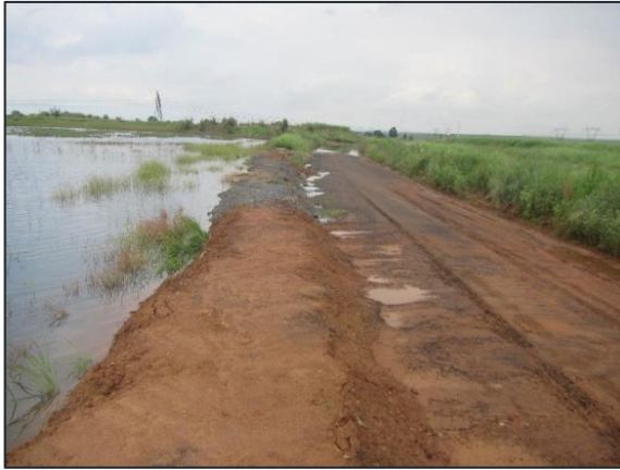
Figure 7-37 - Amongst other features, gravel roads and drainage trenches have fragmented habitat in the local study area, and facilitated alien invasive species colonisation
