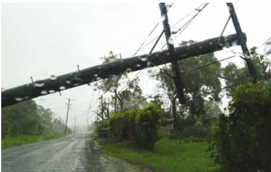
Infrastructure damage after Cyclone Evan, Samoa, 2012
